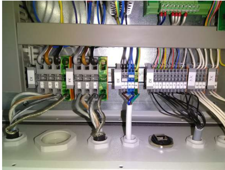
Figure 10: Terminal strip in the control cabinet of the HydroStar counter-current unit (here a double system, in a system with only one turbine the X4 terminals are missing).
